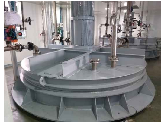
Blenders for the production of petroleum jellies at our Taloja Plant
